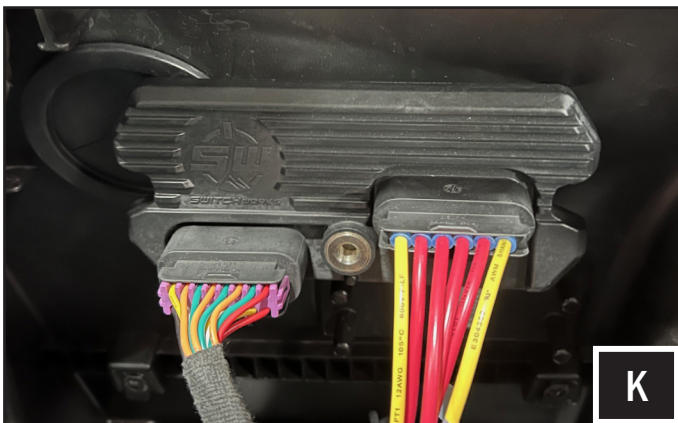
K. Plug in the Power and Switch harness to the 16-pin connector on the RS6 switcher module.
